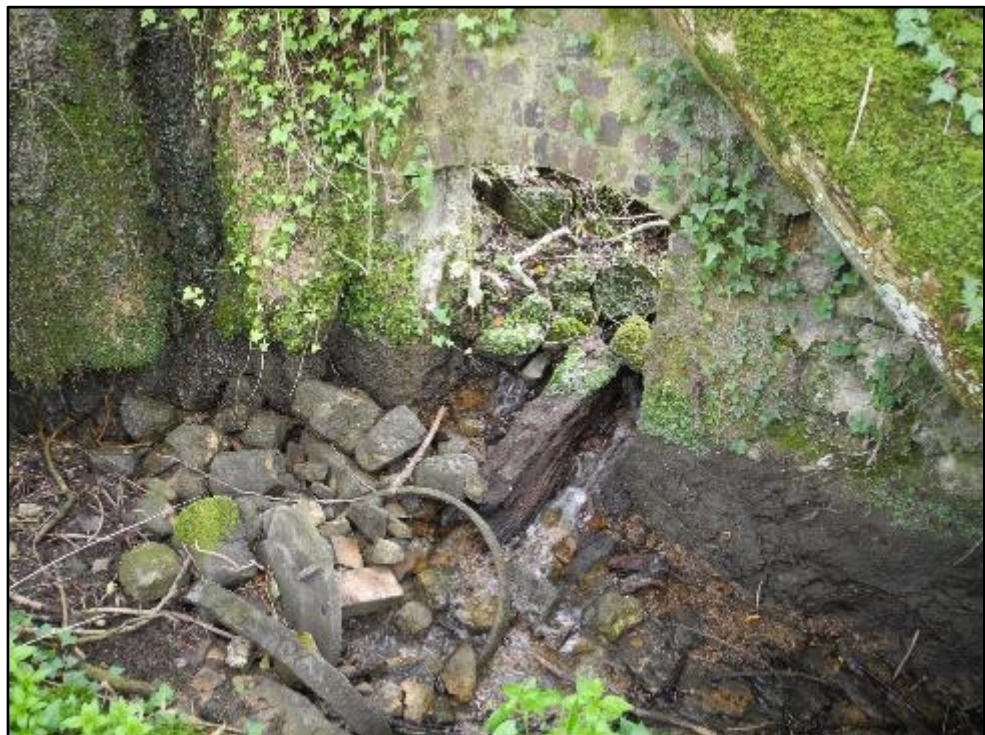
Figure 9 . The base of the wheelpit by the upper buildings. The remnants of the wooden axle can be seen in the arch through to the main buildings. There are also two hoops, which are taken to be strengthening bands around the axle. The end plate of the axle can also be seen with holes suggesting eight arms to the wheel.
